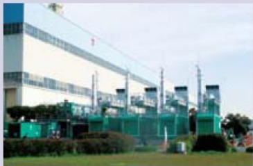
J-Project 5.6 MW PPS in Japan (HYUNDAI - HiMSEN 9H21/32 x 4 Sets)
